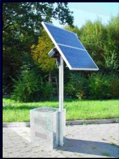
Remote Power Needs
